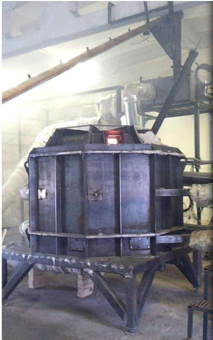
Fig. 3. Combusting chamber of the demonstration plant
